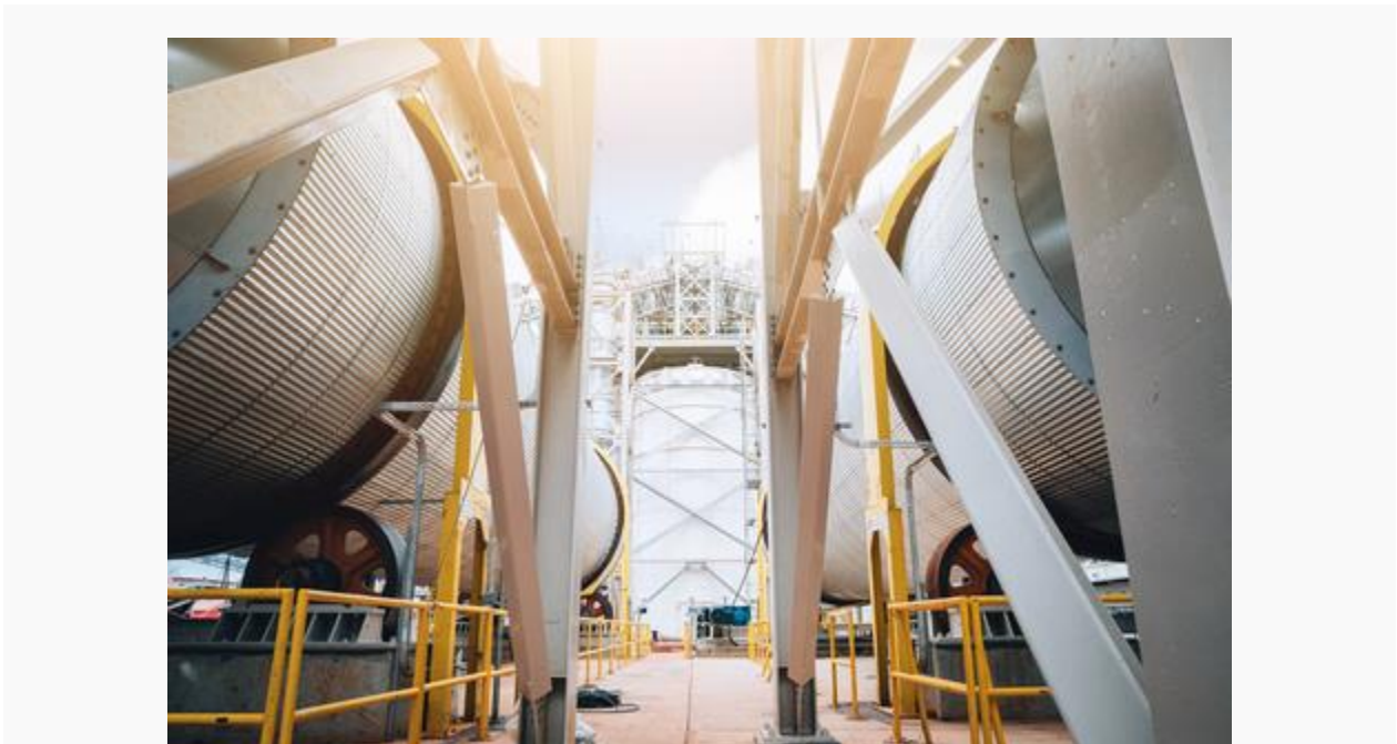
Enviva's recently constructed Lucedale wood pellet manufacturing facility in George County, MS. (Photo: Business Wire)
